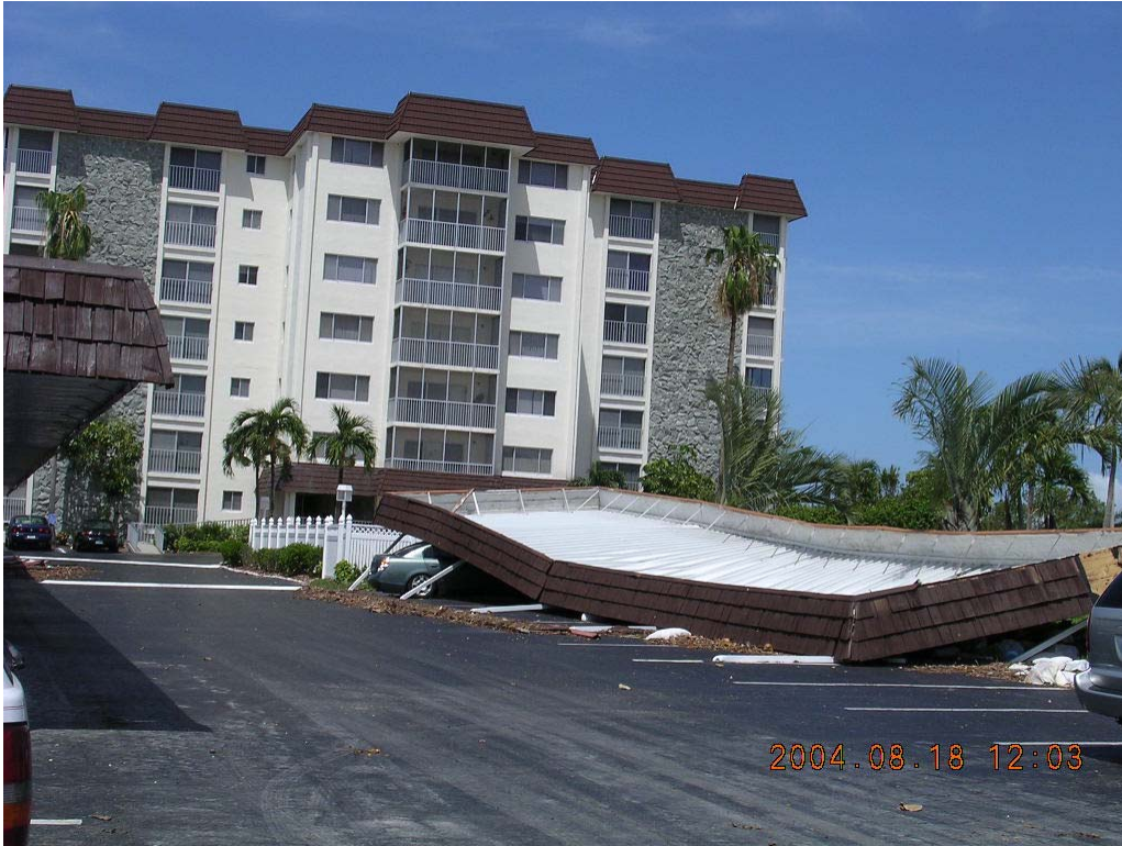
Photo 25. Typical canopied parking structure destroyed (R202)
