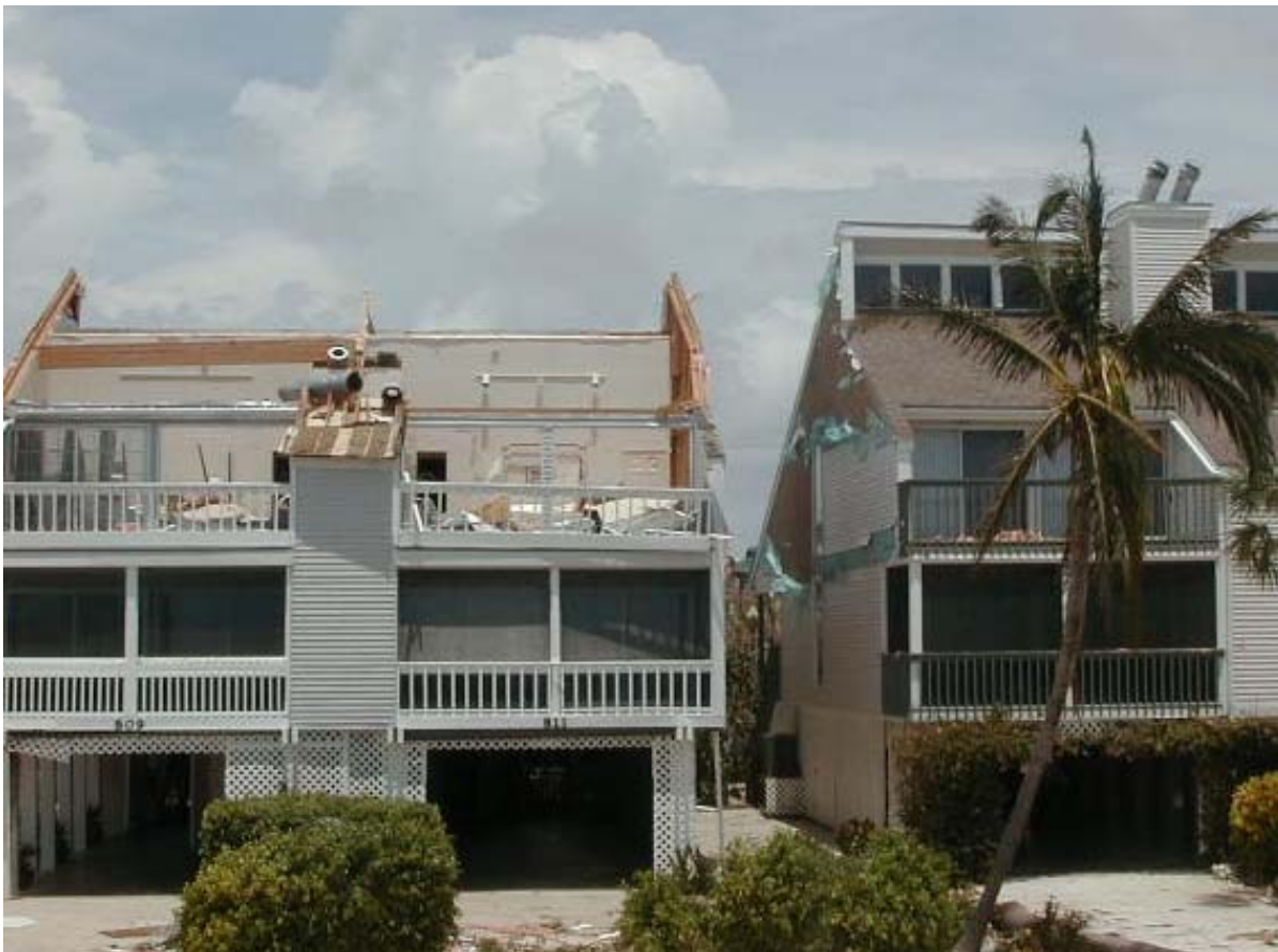
Photo 3. Belcher Road dwelling with roof damage (R25)
