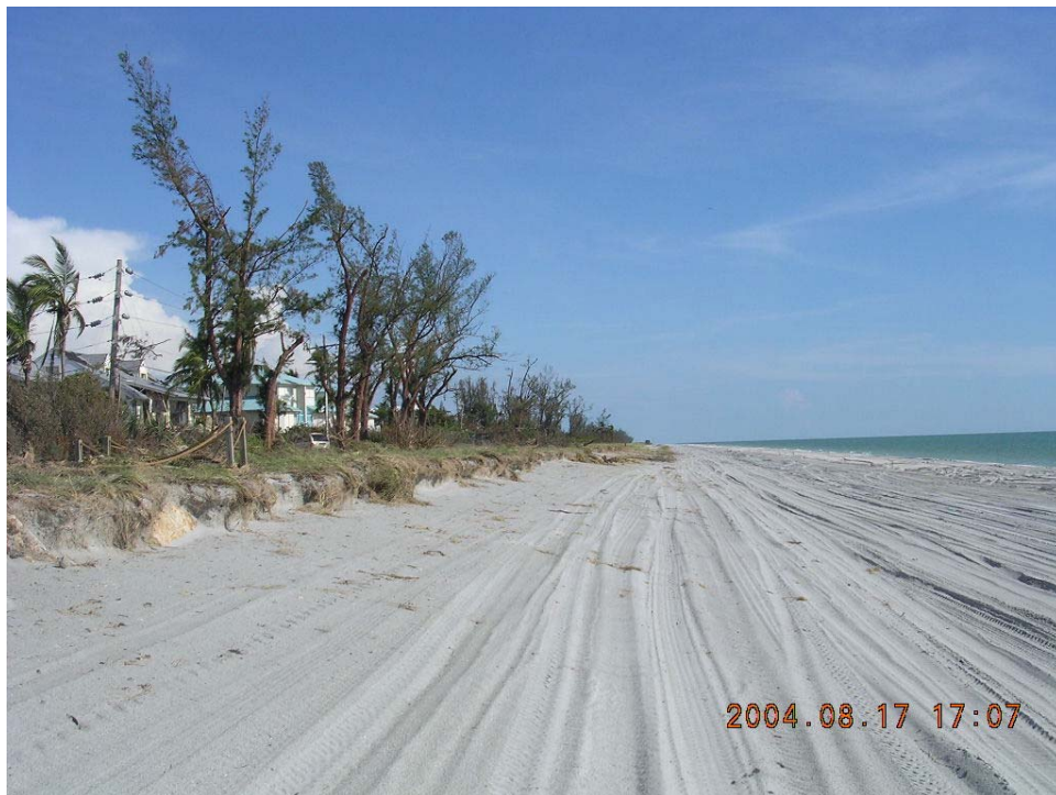
Photo 17. Minor beach and dune erosion, Captiva Island (R97)
