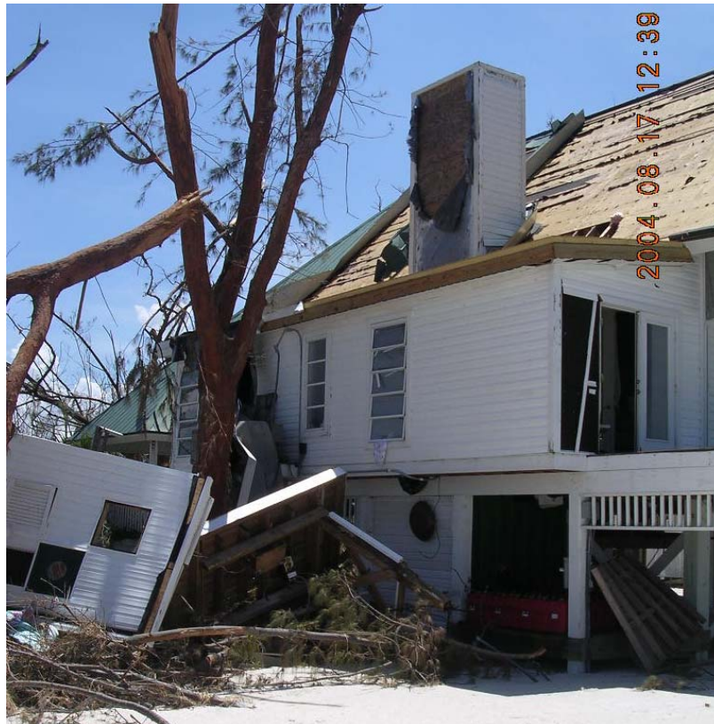
Photo 12. Typical damage at south end of North Captiva Island (R81)
