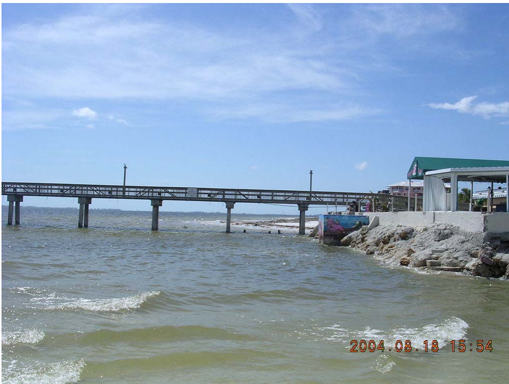
Photo 20. Major beach loss adjacent Ft. Myers Beach Pier (R181)
