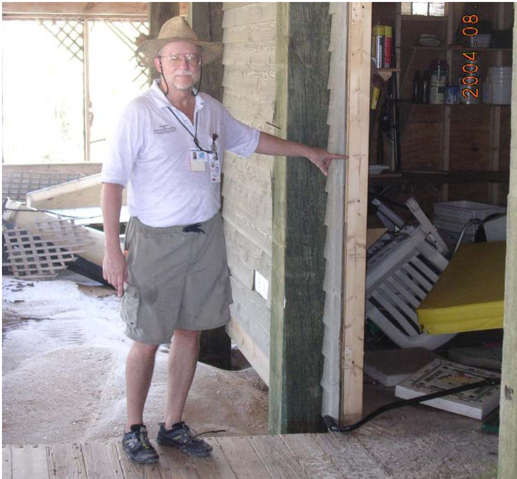
Photo 13. Storm surge elevation of approximately +9 feet on North Captiva Island
