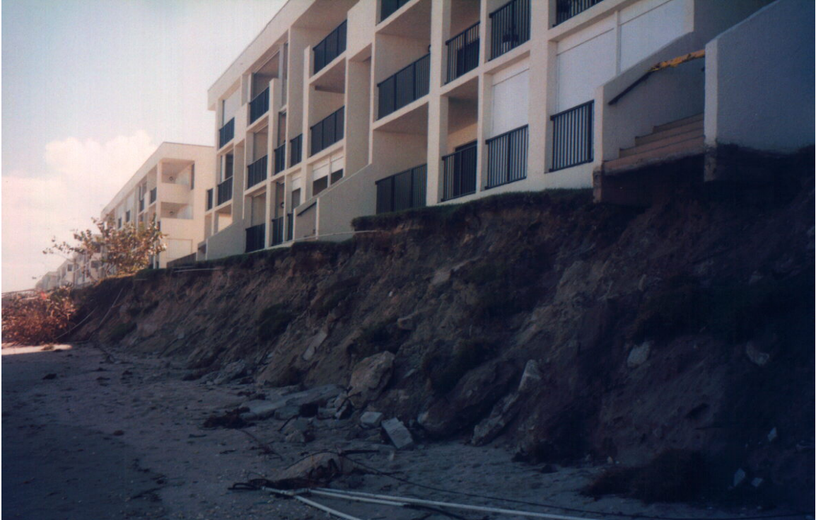
Photo 10. Additional erosion from Irene beginning to undermine threatened buildings.
