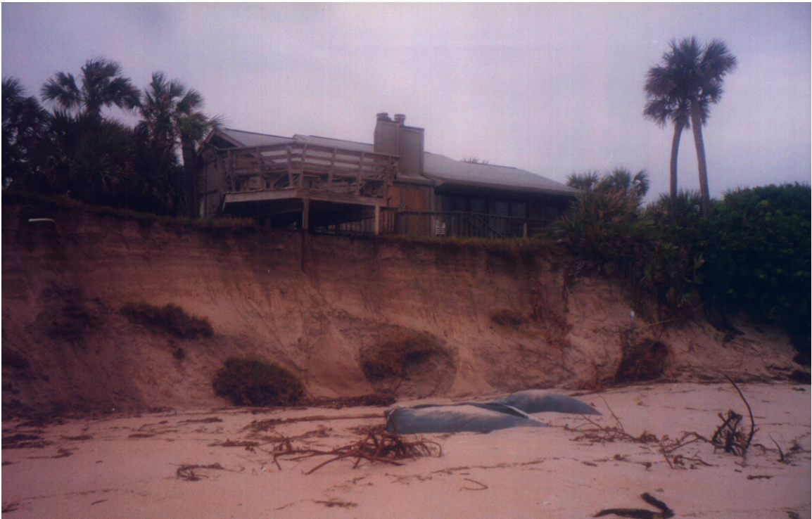
Photo 12. Summerplace Subdivision dwelling threatened by Floyd's erosion.
