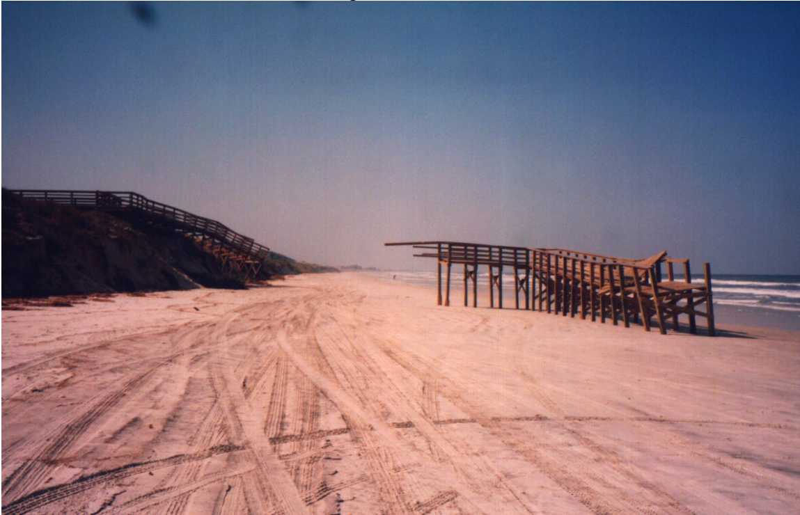
Photo 3. Ft. Matanzas National Monument beach and dune erosion and deck damage.
