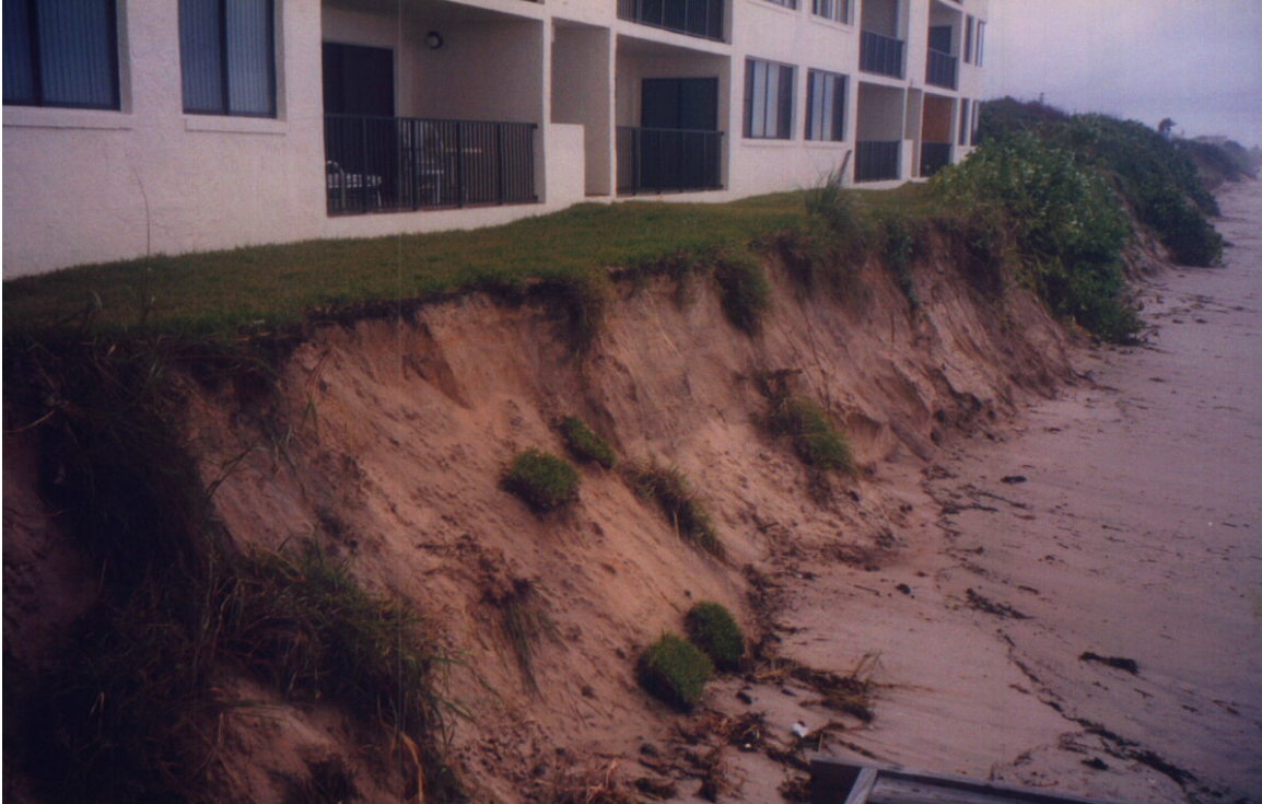
Photo 9. Floyd's erosion at the Breakers Condominium, Melbourne Beach.
