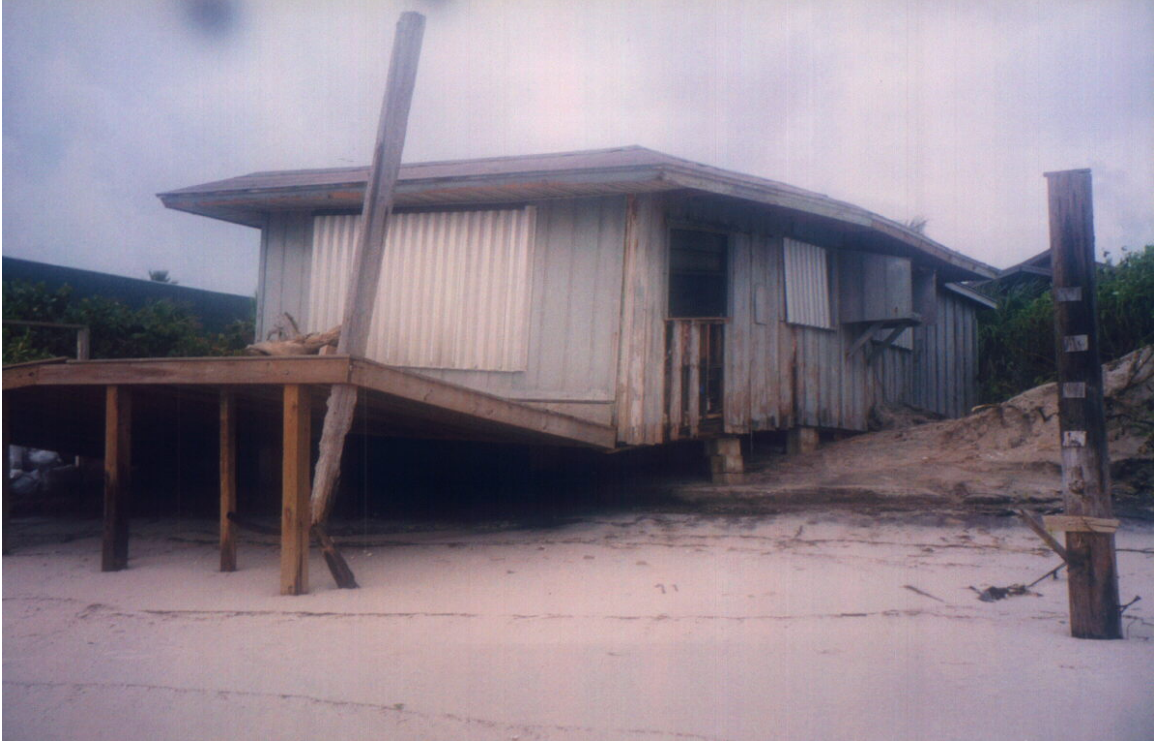
Photo 11. Ambersand Beach dwelling damaged by Floyd.
