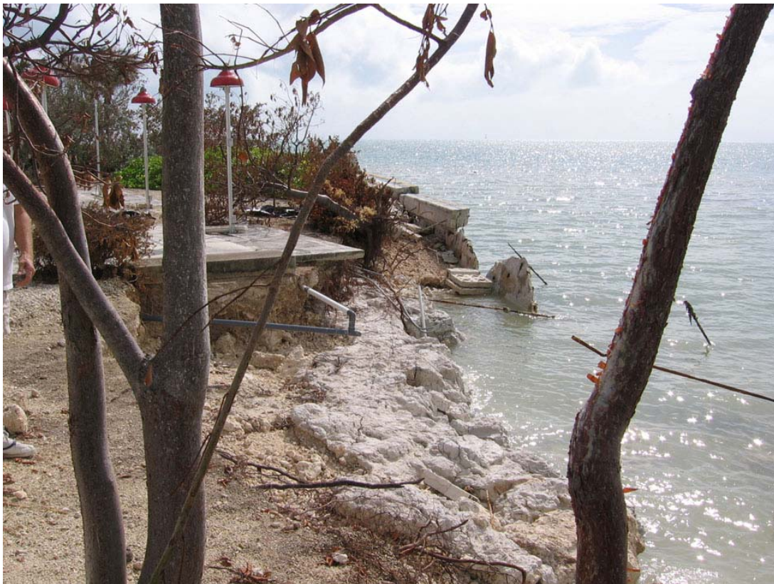
Photo 44. Seawall destroyed by Wilma, Tingler Island.
