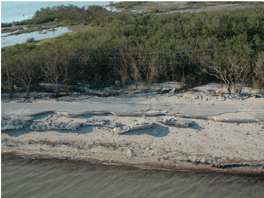
Photo 52. Boca Chica Beach Road damaged.
