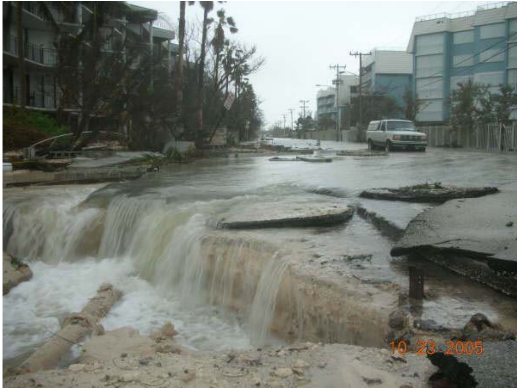
Photo 55. Bertha Street during Wilma's falling storm surge. (Credit: City of Key West)
