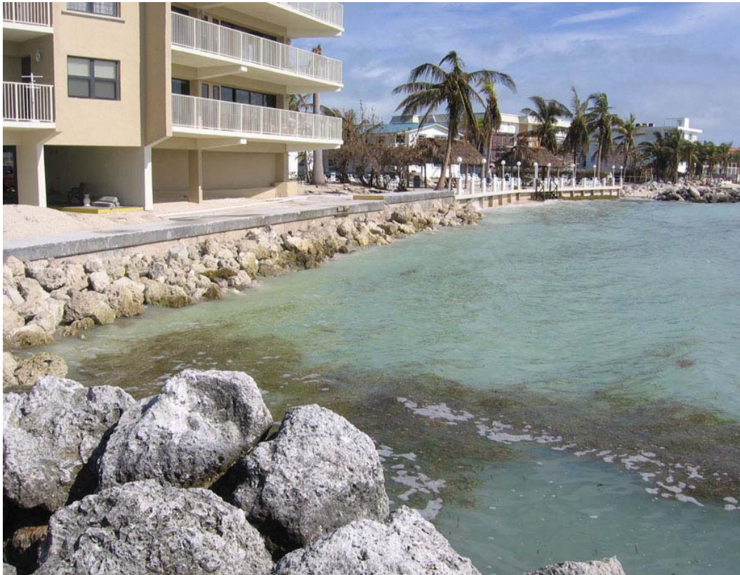
Photo 28. Complete loss of emergent beach at Key Colony Point, Key Colony Beach.
