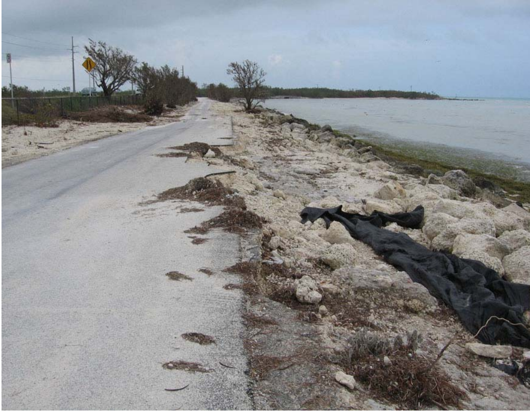
Photo 47. Road and revetment damage, Bahia Honda State Park.
