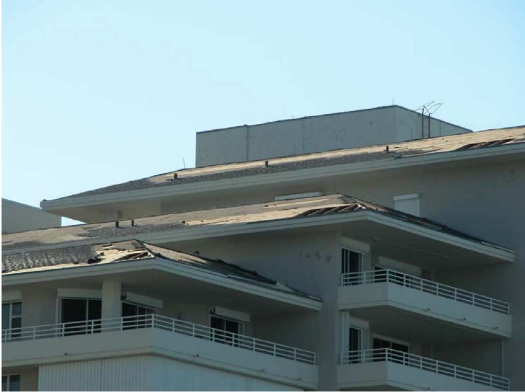
Photo 18. Major roof damage, Marco Island (R145.4).
