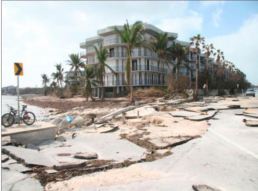
Photo 56. Bertha Street damaged. (Credit: City of Key West)
