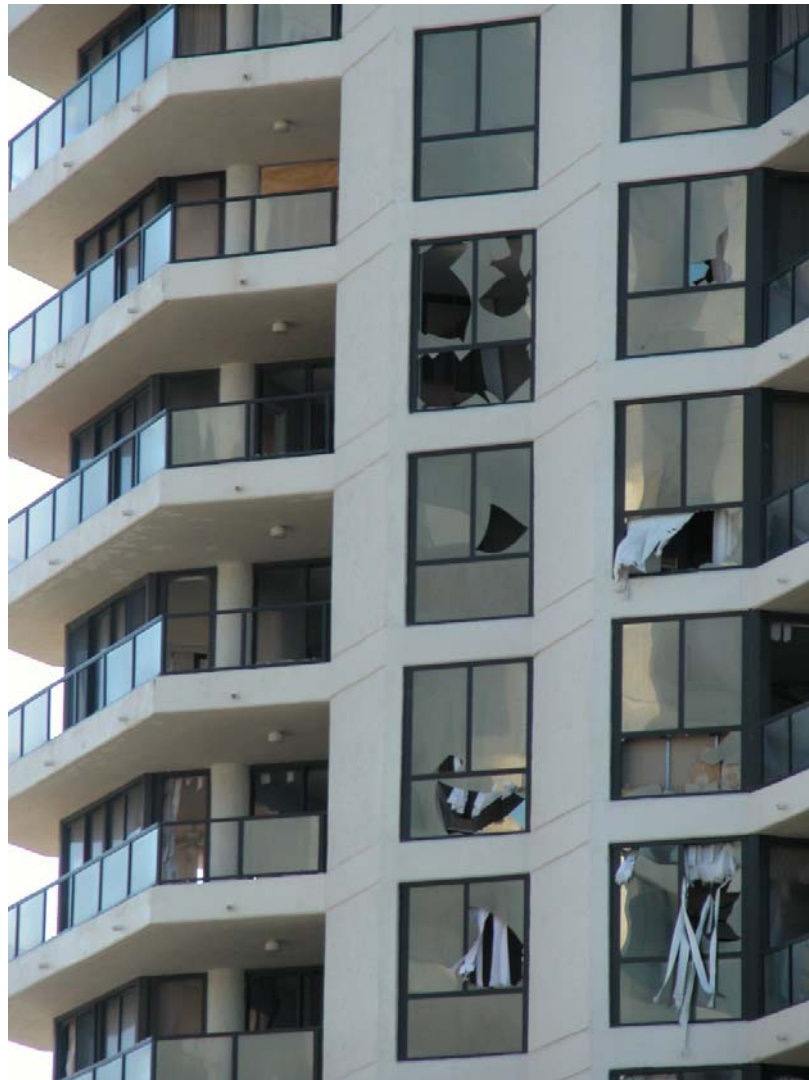
Photo 17. Window damage to high-rise condominium (R145.3).
