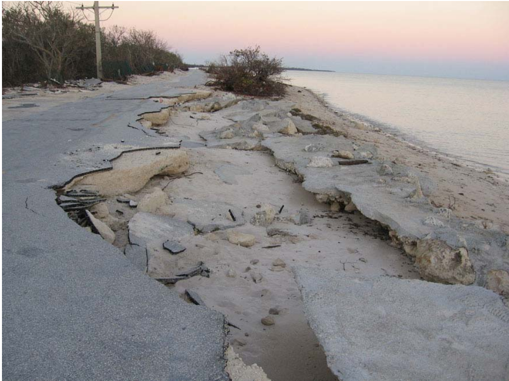
Photo 51. Boca Chica Beach Road damaged.
