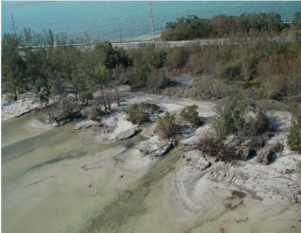
Photo 24. Storm surge scour channels, Long Key State Park.
