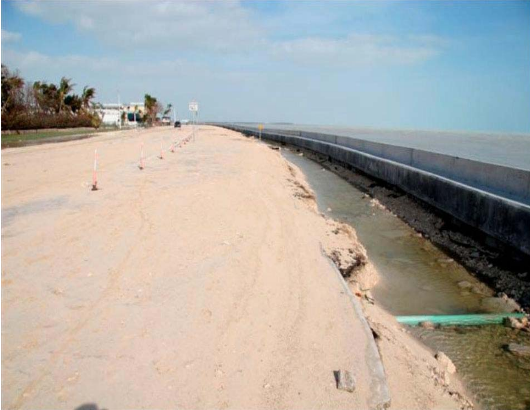
Photo 34. Scour behind seawall along South Roosevelt Boulevard (Credit: City of Key West).
