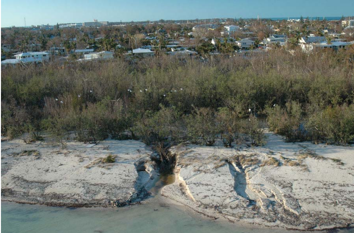
Photo 37. Scour channel, Berg and Kitsos Beach.
