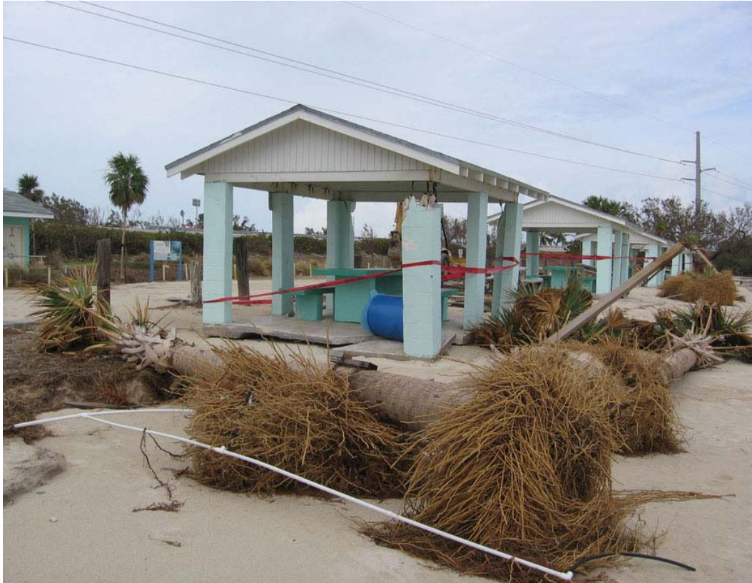
Photo 45. Damaged picnic shelter, Little Duck Key.
